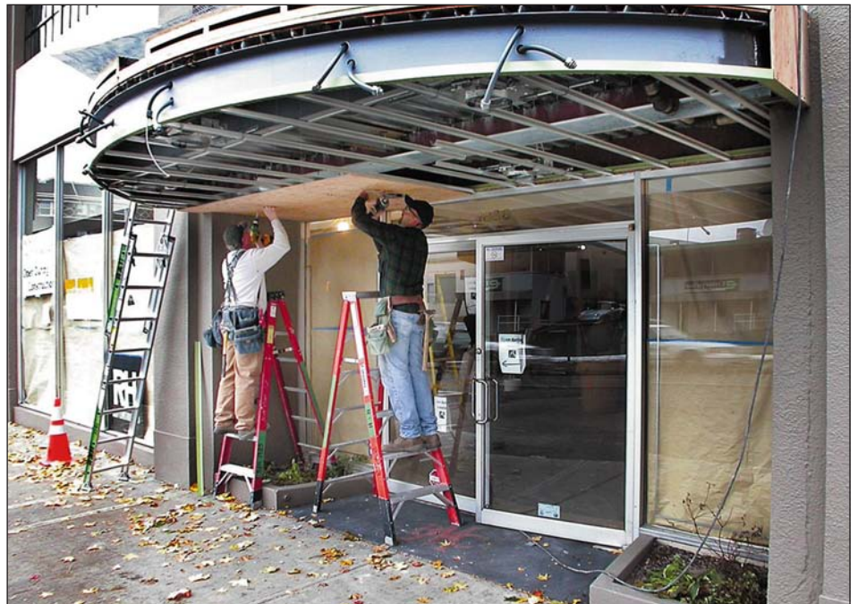
R&H Construction Carpenter Earl Penton (right) and Superintendent Scott Staat work on the new canopy for Monte Shelton Motors on West Burnside Street in Portland. Working with Scott/Edwards Architecture LLP and R&H Construction, the Portland firm of Bainbridge Design is not only serving as project manager for the design team but project manager for the construction as well.
